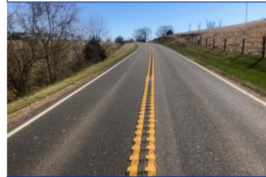
Centerline Rumble Strips
